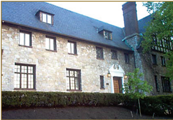
The house in May 2005, with new windows on the second and third floors.
